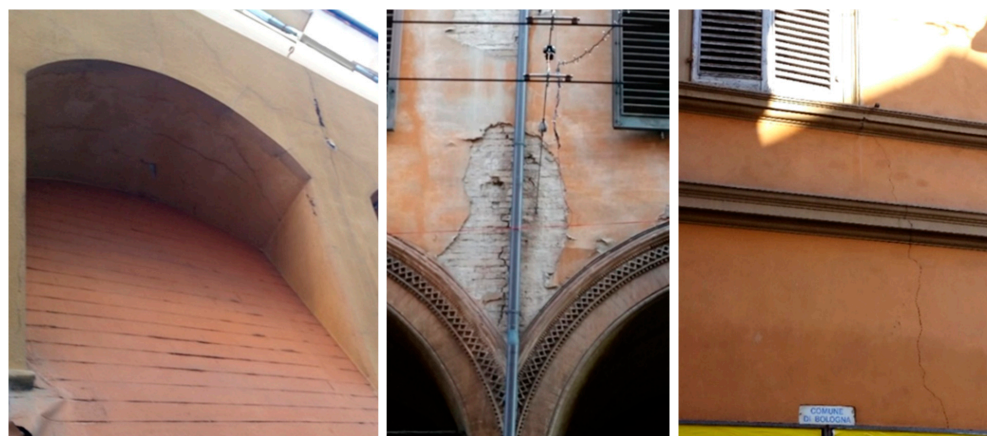
Figure 13. Typical cracking patterns due to gravity loads and lack of tension resistance and load distribution, Bologna, Italy.
