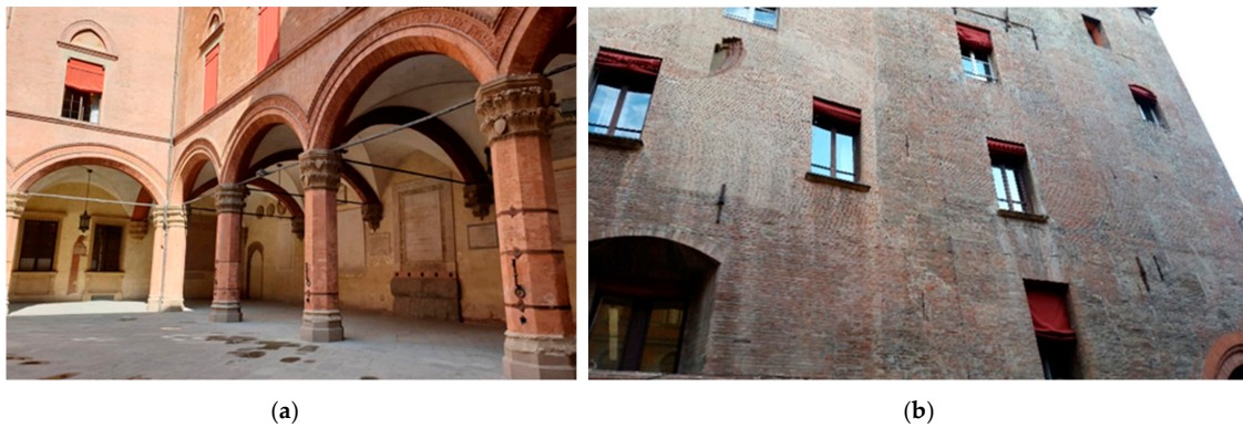
Figure 12. (a) A coupled system of cross vaults reinforced by steel tie rods; (b) reinforcement by steel tie-rod and bar-shaped anchor plate, Bologna, Italy.
