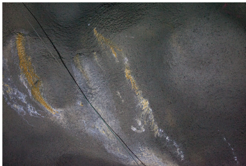
Figure 5. Examples of leaching of the shotcrete in a hard rock tunnel, from Sjölander and Ansell [1].
