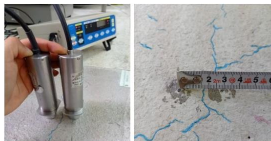
Figure 12. The crack depth measurement process using an ultrasound device.
