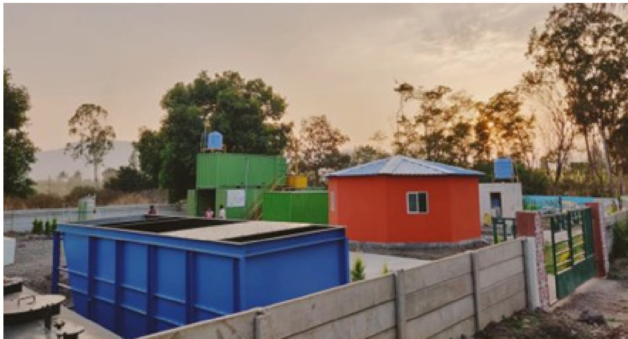
Figure 2. Photo of the community scale faecal sludge and septage treatment plant in Wai, Maharashtra (Tide Technocrats, n.d.)
