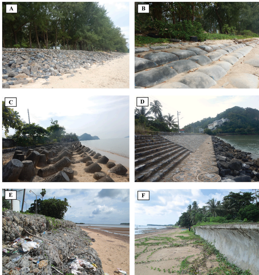
Fig. 2. Different types of revetment. (A) A rock revetment, (B) a sandbag revetment, (C) a concrete tetrapod revetment, (D) a grouted rock revetment, (E) a gabion revetment, and (F) a curve-faced concrete revetment.
