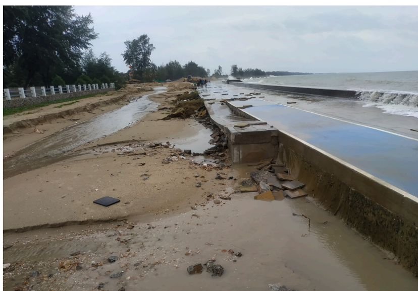
Fig. 8. The retained water damaged the facilities on a revetment crest.
