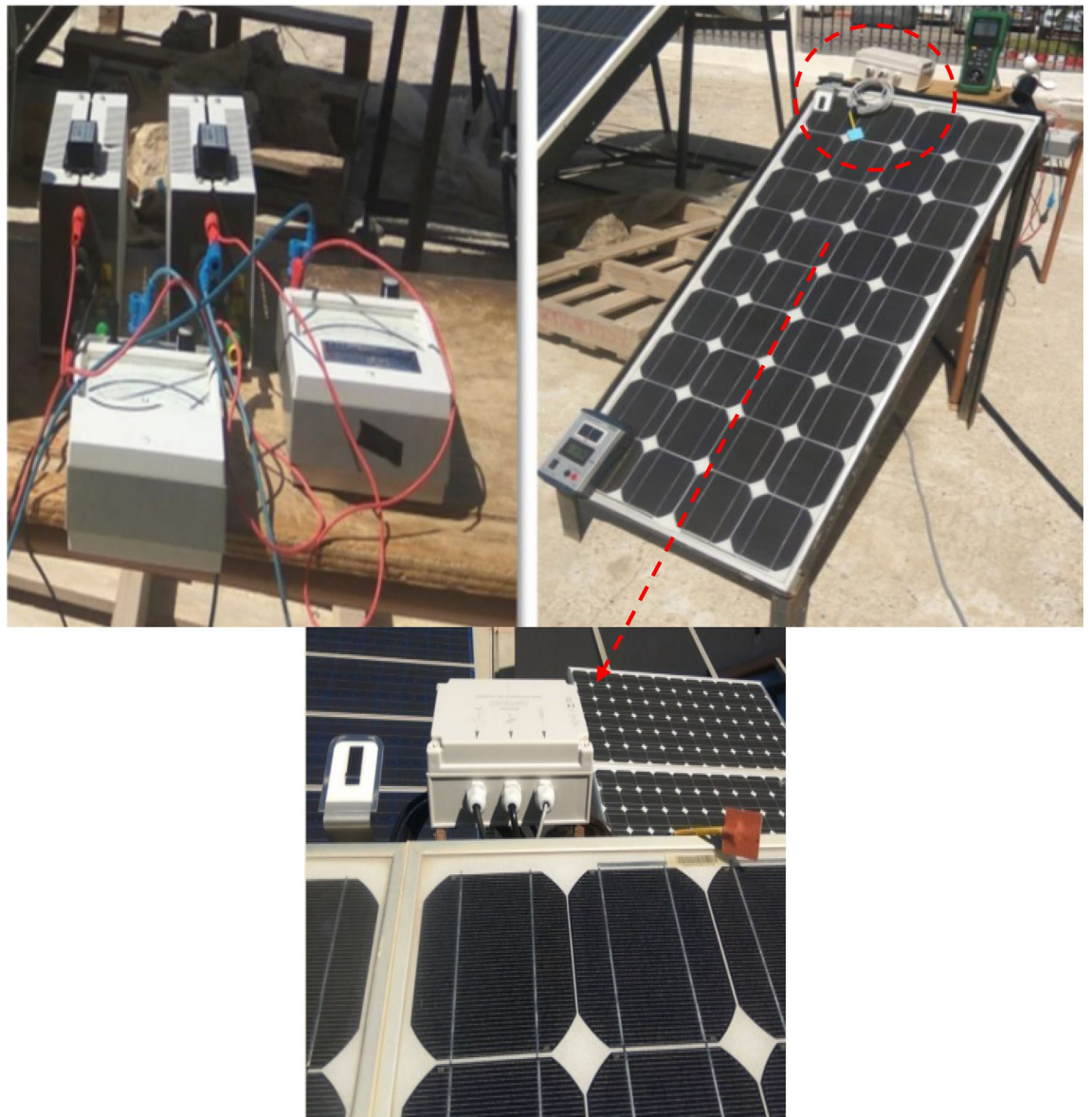
Figure 3. Determination of the electrical characteristics.
