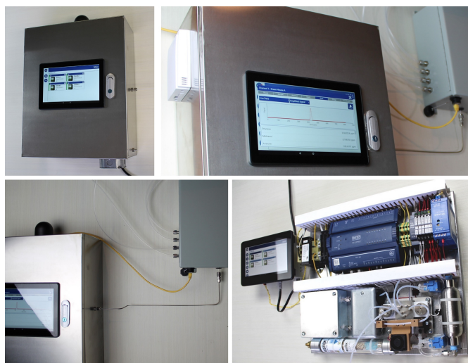
Figure 10. Industrial-grade compact Adelphi ethylene/VOC monitor based on a DISTECH controller.
