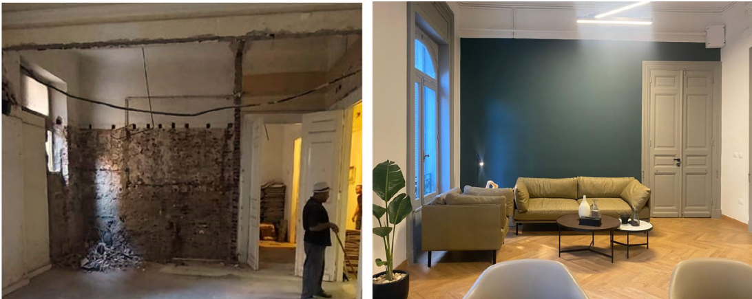
Figure 12. Before and after photos of what currently is a meeting room; the previous tenant destroyed the original window and created a wall in its place. Transgressions were removed and a new window replicating the original design was added once again. Source: This figure has been reproduced with permission from Sigma Properties, 2022.
