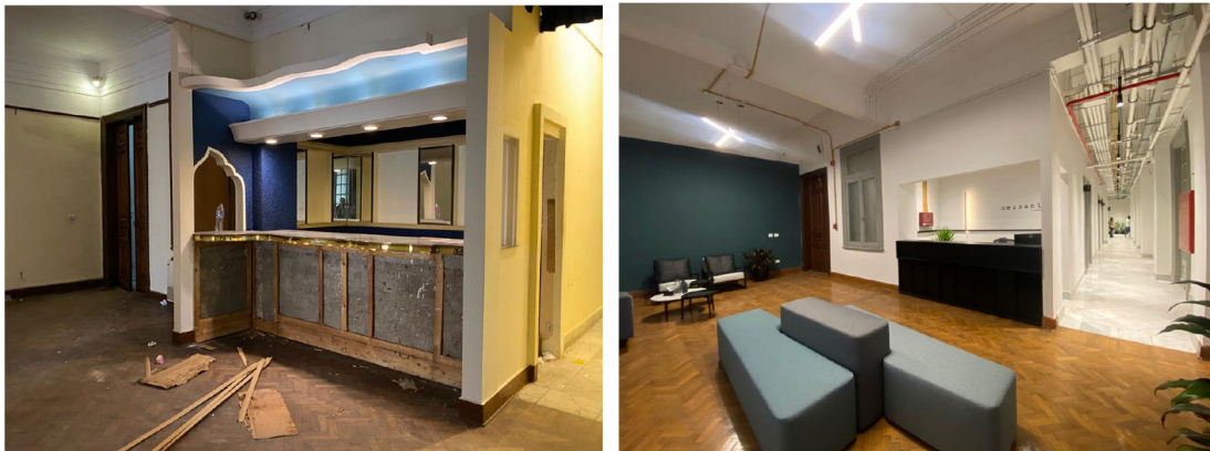
Figure 10. Before and after status of the reception area of the project, the original parquet floors were restored and the existing features were maintained. Electrical systems were installed in an exposed manner in order to preserve the vast heights of the interior spaces. Source: This figure has been reproduced with permission from Sigma Properties, 2022.
