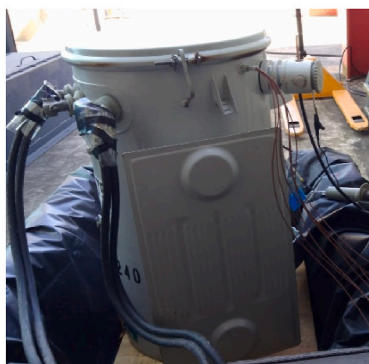
Fig. A1. Instrumented 75kVA single-phase transformer, prior to experiments.
