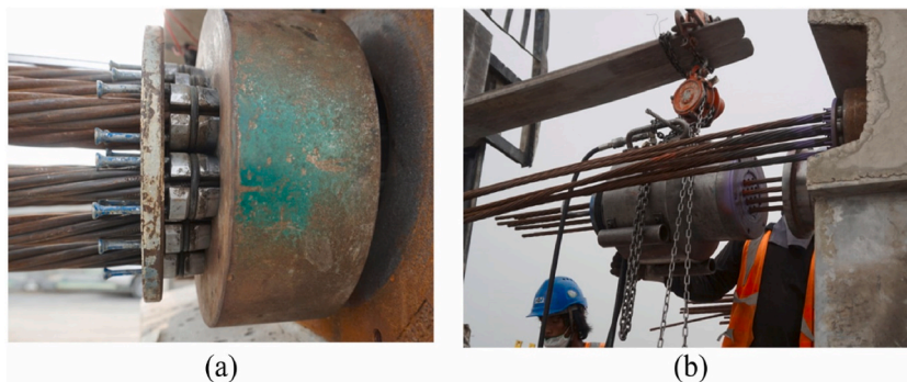
Fig. 2. Post-tensioned concrete in the field: (a) Steel plate and grips and (b) post-tensioning process using a hydraulic jack [70,71].
