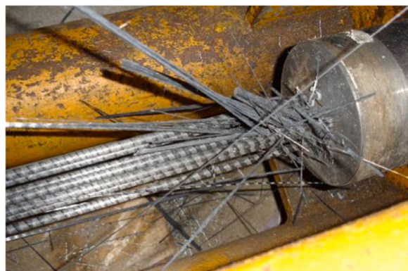
Fig. 10. A typical CFRP tendon rupture [137].
