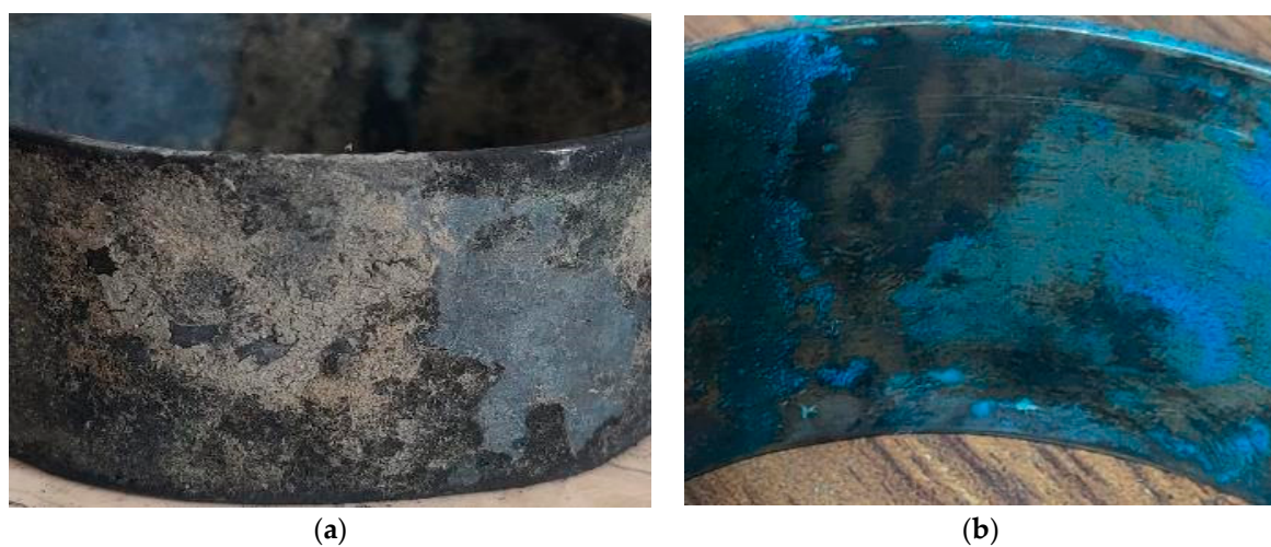
Figure 8. Macroscopic view of corroded coupons of Cu-Ni 90/10 material collected from (a) polluted seawater site and (b) natural seawater site.
