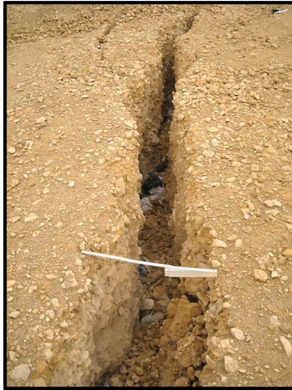
Fig. 8. A half-meter wide tensional cracks developed in the debris deposits, and exhibits no vertical displacement.
