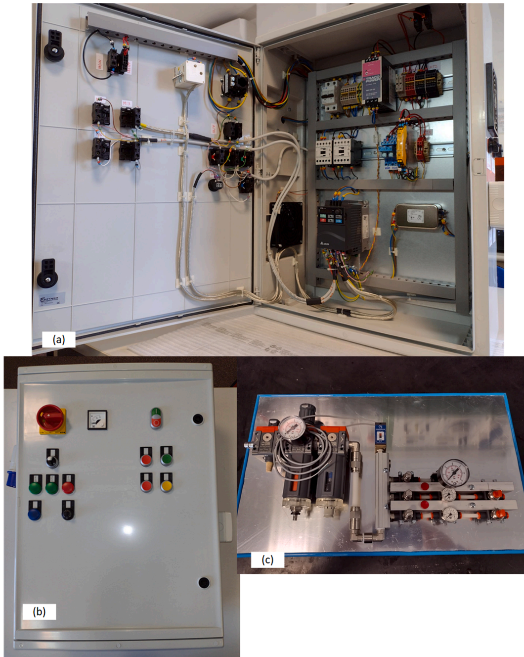
Fig. 23. Picture of the Internal View of the Electrical Cabinet (a), External Front View (b) and the Pneumatic Panel (c).
