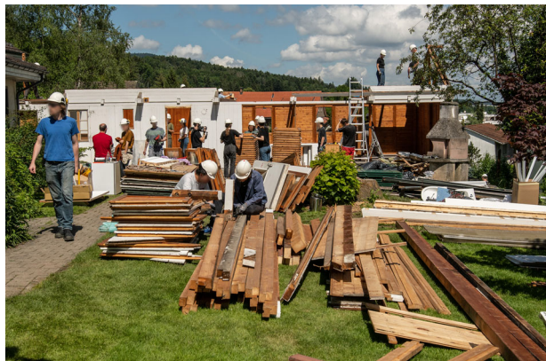
Fig. 5 | Disassembly of the Zurich music pavilion, after scanning and material identification, enabled the cataloguing and sorting of the materials, carried out by the authors in collaboration with industry practitioners and academic students (Photography: Buser Hill Photography).
