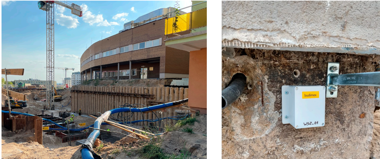
Figure 31. Construction of the Trauma Center of the Regional Specialized Hospital in Olsztyn (Poland); event recorder module installed on the wall of the hospital building adjacent to the construction site.
