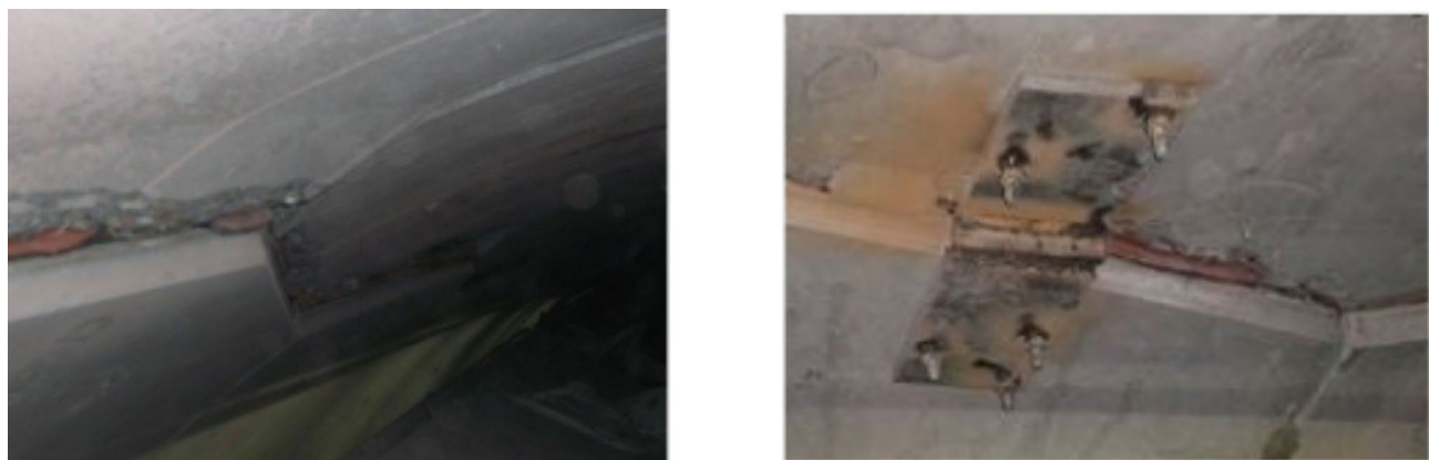
Fig. 6. Deformation of segment on site.
