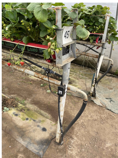
Figure 3. Flow meter inside tunnel.
