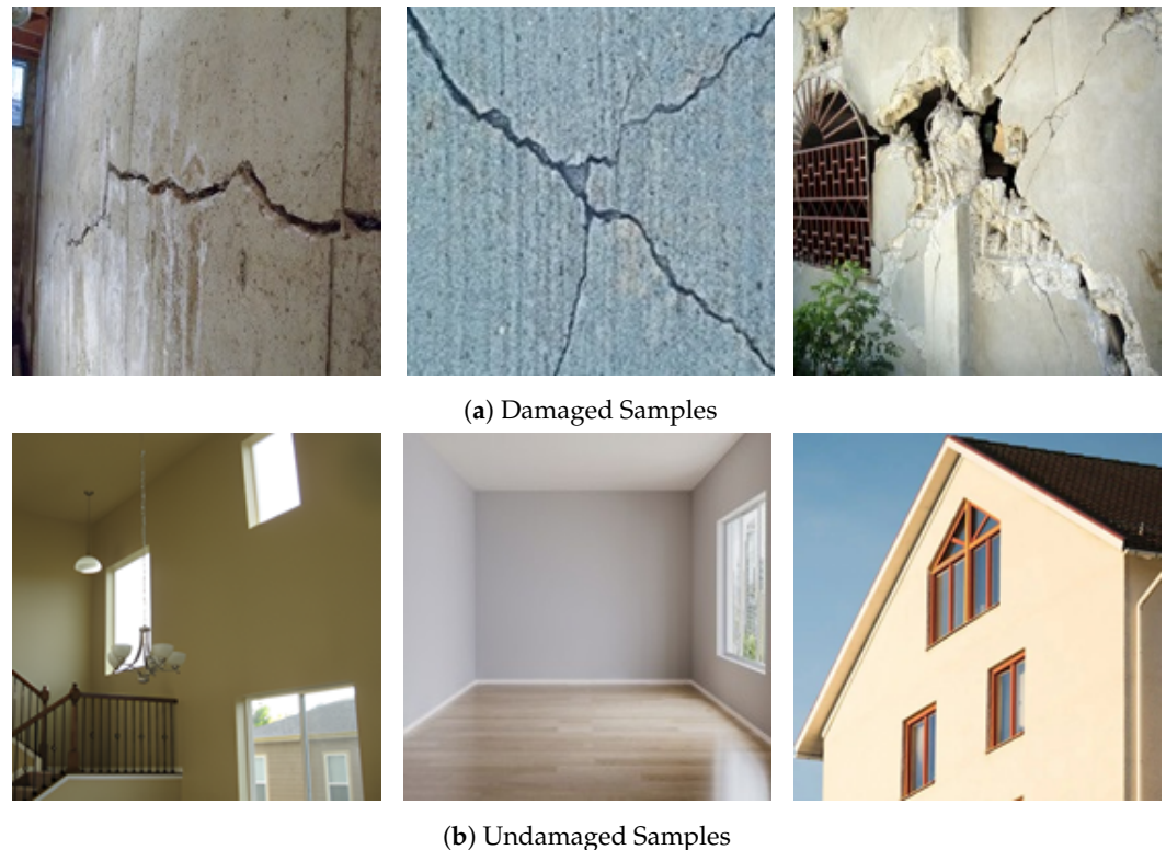
Figure 9. Samples of (a) damaged structures and (b) undamaged structures.
