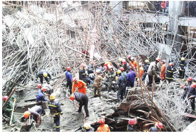
Fig. 1. Collapse accident of the high-formwork support frame.
