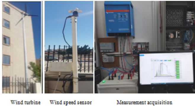
Fig. 4. Measurement acquisition device at the laboratory.
