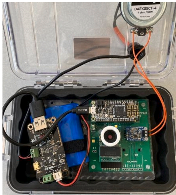
Fig. 20. Shows added solar charge controller.
