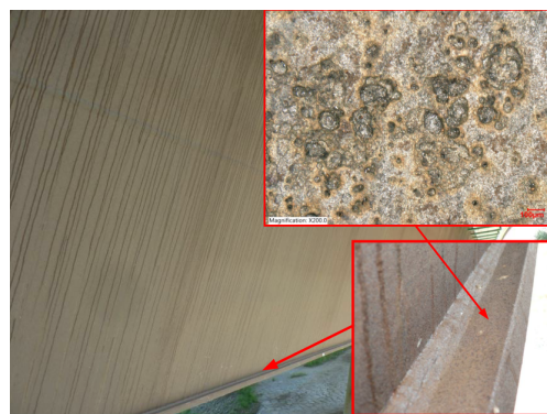
Figure 16. Bridge across the Ostravice river, Czech Republic; photo and detail of the connection of the exterior web plate and bottom slab plate of the box girder; the top surface of the bottom slab of the bridge—magnification 200×, Keyence VHX-7000.
