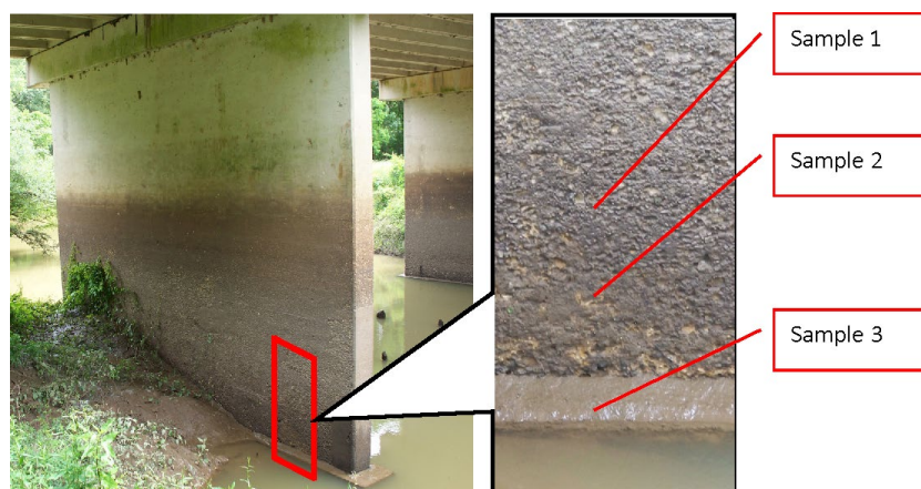
Figure 4. The concrete samples from a bridge site in Texas. Reproduced with permission from Trejo et al. [27].
