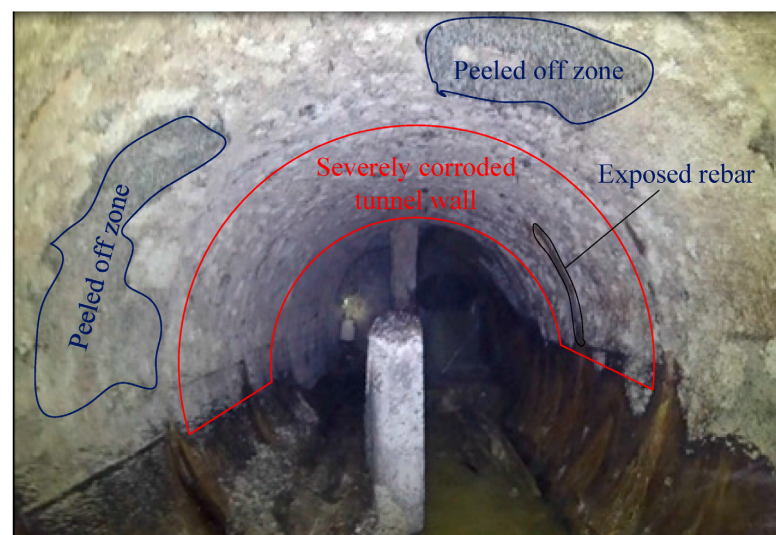
Figure 6. Corrosion conditions in a chamber located under 127 Street and 153 Avenue in Edmonton, Canada. Reproduced from Wu et al. [34]. © 2018 by the authors. Licensee: MDPI, Basel, Switzerland.
