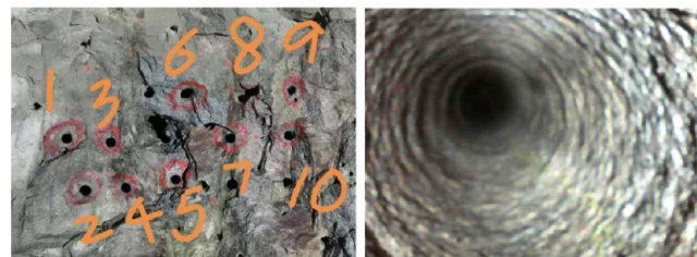
(b) Holes for overall testing of granite layers (c) Granite overall drilling inner edge surface
