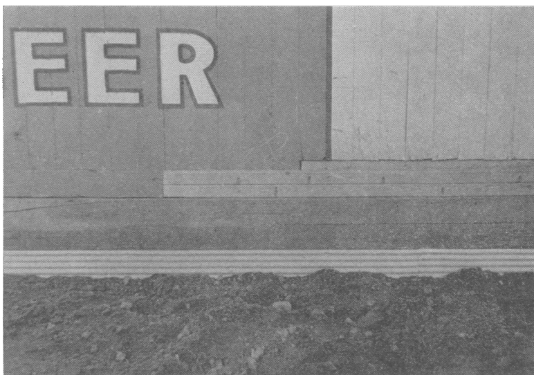
FIGURE 4—Another view of the building in FIGURE 3. A trench 2 feet deep has been dug around the building and a wall of galvanized iron roofing installed 2 feet below the ground level and several inches above. The top edge has been firmly nailed to the building.
