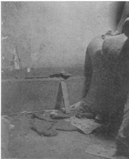
FIGURE I—Example of structural rat harborage existing in the enclosed spaces formed by double walls and raised flooring
