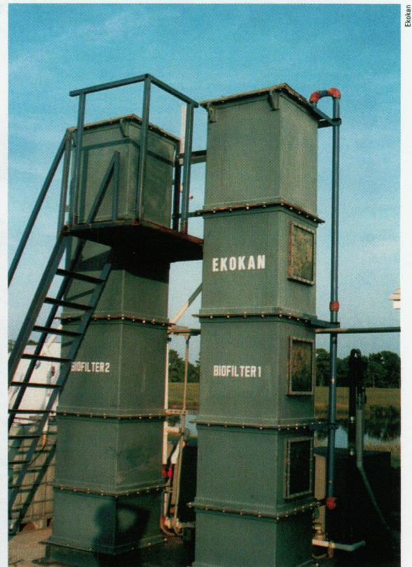
Twin towers. Waste separators in which odorous compounds are broken down by bacteria are another promising technology.
