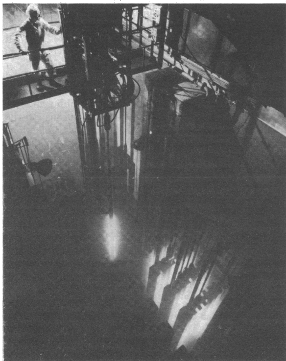
FIG 2—Fuel storage pond, steam-generating heavy water reactor, AEE Winfrith, Dorset: Cerenkov radiation from irradiated fuel. (Reproduced by courtesy of the United Kingdom Atomic Energy Authority.)
