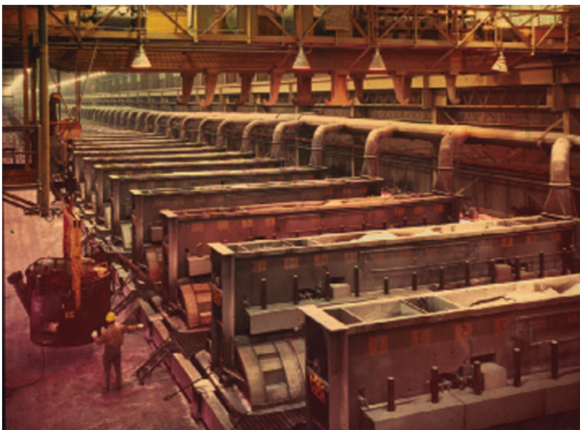
Figure 5 Fume extraction system in a pre-bake potroom.
