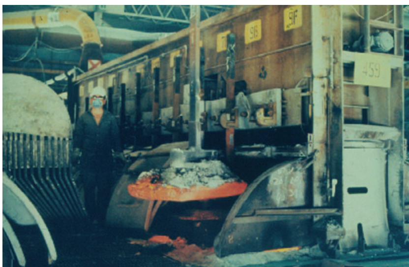
Figure 3 Removal of a spent anode in a pre-bake potroom.
