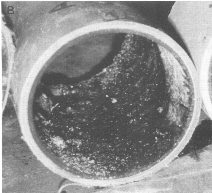
FIG. 3. Pipes coated by CCS after 374 days with no applied potential (A) and with a potential of 1.2 V versus the SCE (B). The experimental period was 1 August 1990 to 7 August 1991, and the seawater flow rate was 0.53 m/s.
