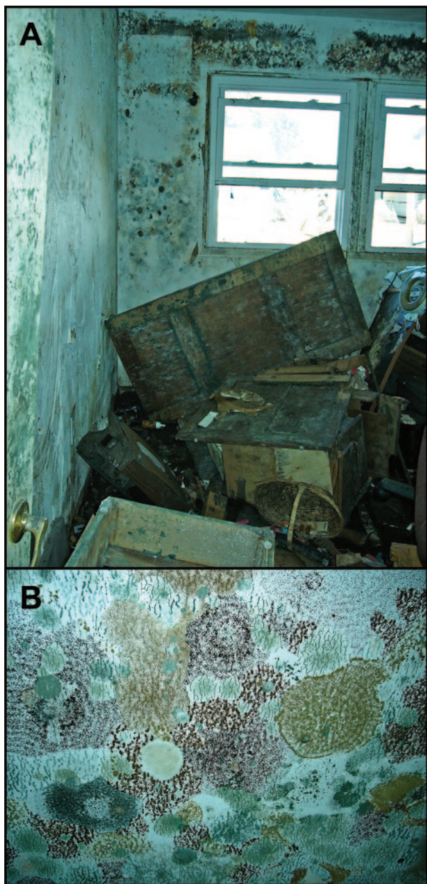
FIG. 1. Visible mold and damage in a bedroom (A) and on the ceiling (B) of a representative house in St. Bernard's Parish on 10 October 2005.
