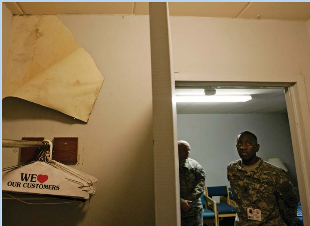
Bad scene. A section of wallpaper is pulled back to reveal mold in Building 18 of the Walter Reed Army Medical Center. Indoor mold and the bacteria that often grow with it are believed to pose a greater threat to immunocompromised people.
