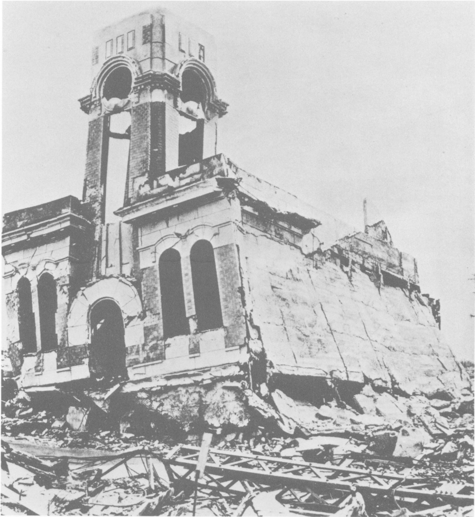
Figure 1 —A building 0.4 mile from ground zero at Hiroshima. The walls were constructed of reinforced concrete.
