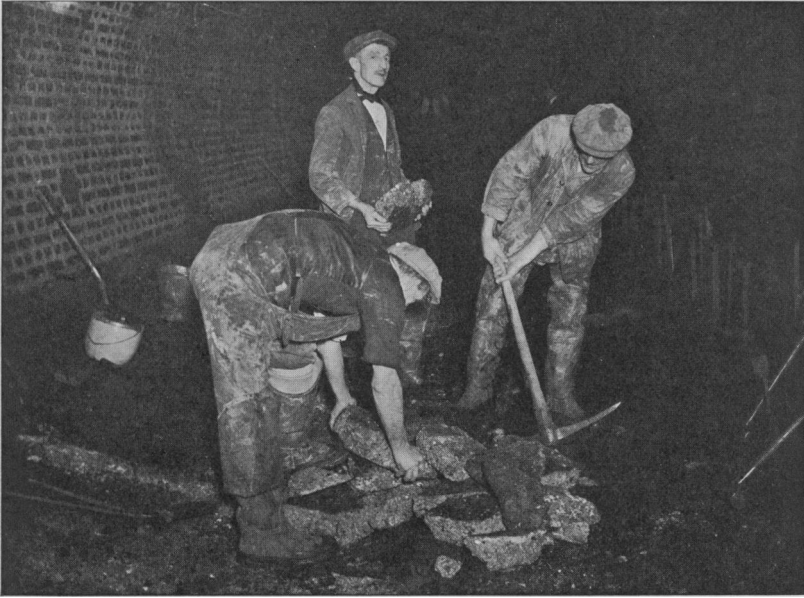
FIG. 1. —Showing builder's labourers breaking the floor of a sewer and removing by hand pieces of slime-covered concrete.
