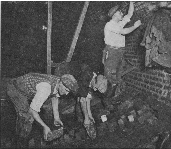
FIG. 2. —Showing men handling the broken concrete beside the new brick-work by which it is being replaced.
