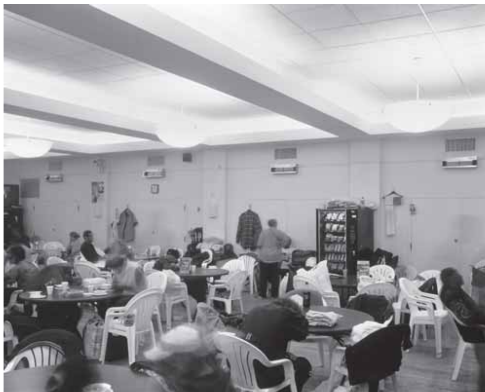
Tuberculosis Ultraviolet Shelter Study New York City shelter in a church basement. Note the ultraviolet germicidal irradiation fixtures located on the upper wall, directly below the vents. Photo: ©Randall Perry Photography.
