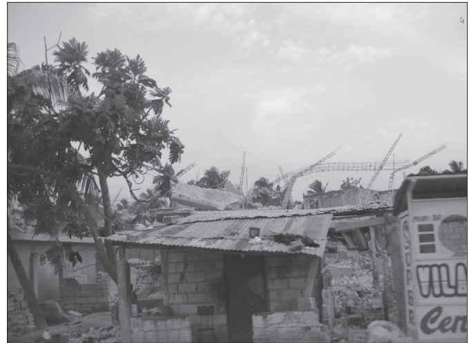
Figure 1. A building damaged through the Haitian earthquake of January 2010.
