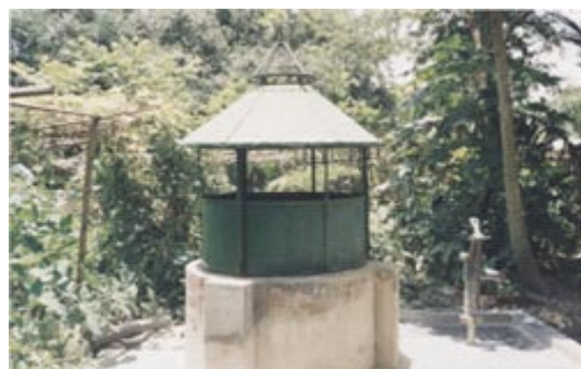
Fig. 5. Water-tank from which gravity feeds the houses
