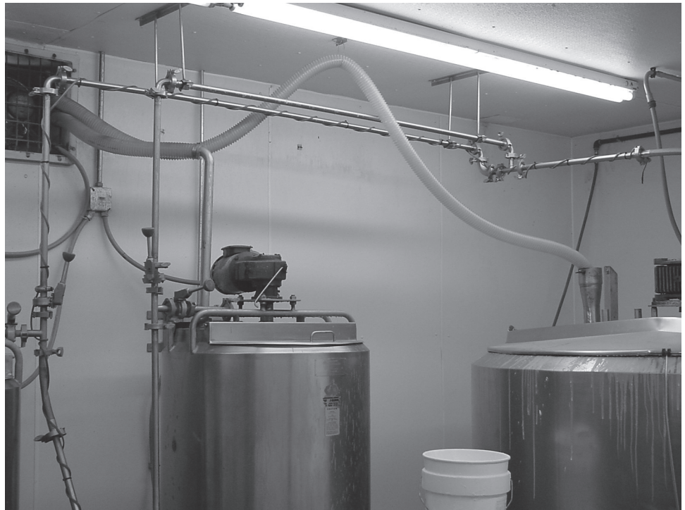
Photo 4: Mixing room after implementation of exposure controls shows exhaust fan on wall and local exhaust ventilation hoses on tanks. Courtesy of the National Institute for Occupational Safety and Health.
