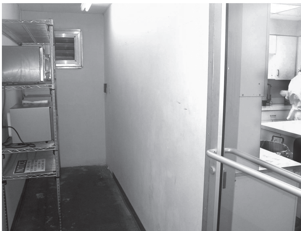
Photo 11: Microwave ovens in new “popping room” with additional exhaust ventilation. Courtesy of the National Institute for Occupational Safety and Health.
