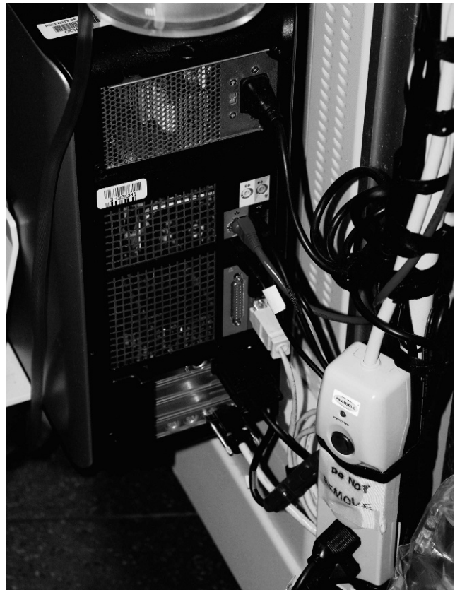
Figure 8. Multiple cables at the back of the DocuSys computer.
