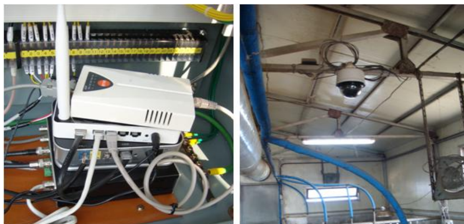
Figure 13. DVR and CCTV.
