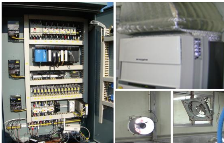
Figure 14. Digital Controller (PLC) and Hog Farm Facilities.
