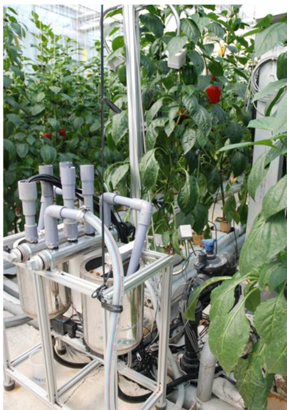
(e) Watering System
