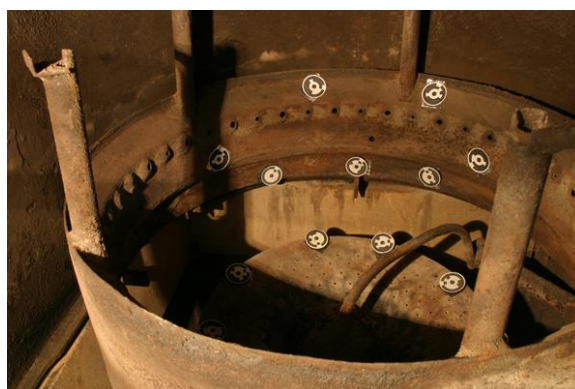
Figure 5. Boiler with coded targets.
