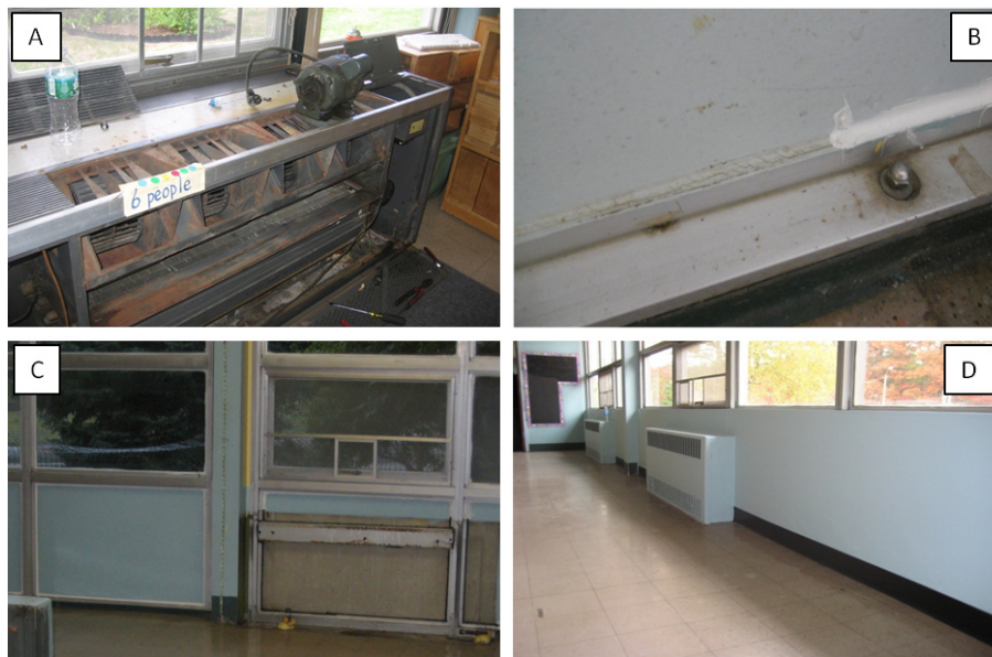
Figure 1 Photographs of interventions: A) unit ventilator with cover and fan motor removed; B) detail of PCB caulk in original and encapsulated form; C) curtain wall with PCB caulk directly accessible to room (left side) and located behind a convective heater that was removed (right side); D) finished false wall constructed over encapsulated PCB caulk, transite panels, and aluminum framing.
