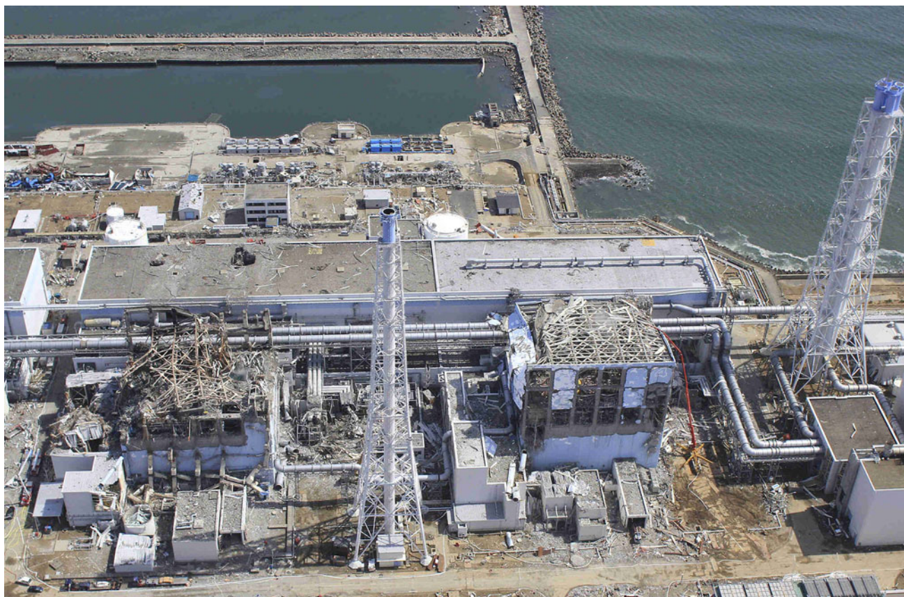
Fig. 15 Damage to the reactor buildings of units 3 and 4 caused by hydrogen explosions on March 14–15 (NAIIC 2012). It is assumed that hydrogen from unit 3 leaked into unit 4 via common ventilation ducts. Photo: Air Photo Services, Japan
