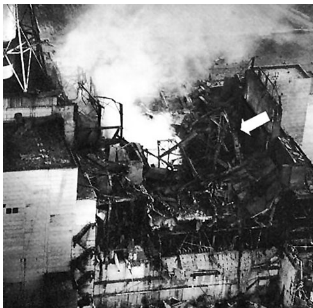
Fig. 9 The damaged and burning core region of the Chernobyl-4 reactor in the first days after the accident. The arrow points to the overturned 1000 ton lid of the core cavity. Photo: Unknown Soviet photographer
