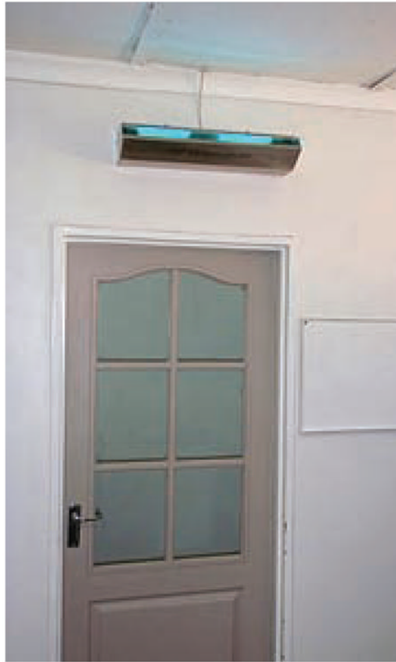
Figure 6. Upper room ultraviolet germicidal irradiation fixture.
