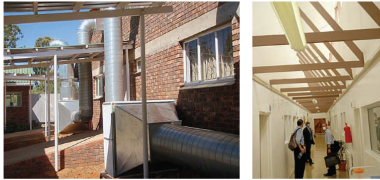
Figure 4. Lesotho, with simple mechanical ventilation system, maintained by a service contract, and separation and isolation capacity.
