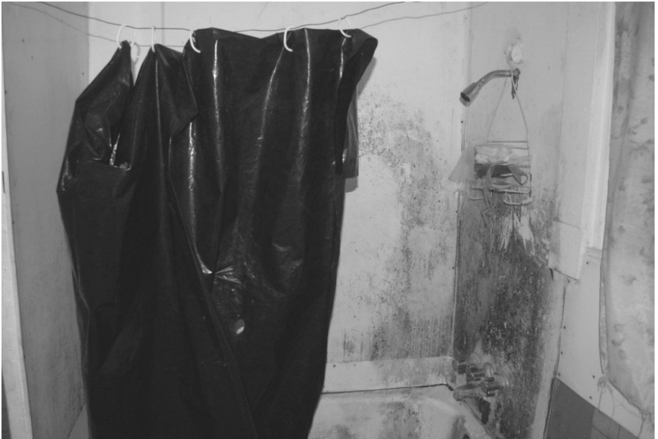
Figure 2. Migrant farmworker shower showing accumulation of mold, Eastern North Carolina, 2010.
