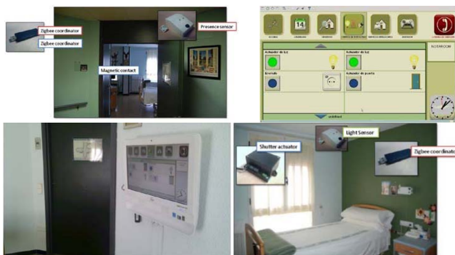
Figure 5. LSFT installation: The pictures show some of the sensors integrated into the LSFT as well as the Human Machine Interface in the rooms.
