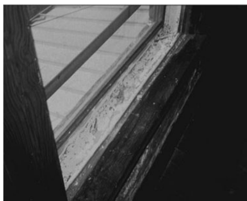
Fig. 1 Typical deteriorated lead-containing paint from inner city housing identified in home visit for TLC study [used with permission of Walter Rogan MD]
