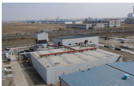
FIGURE 9: Full-scale 11,000 kg-N/d one-step ANAMMOX installation at the Tongliao Meihua Company in China, Courtesy Paques [121].
