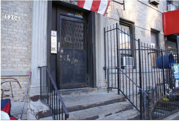
FIGURE 1: The offending door and stair railing.
